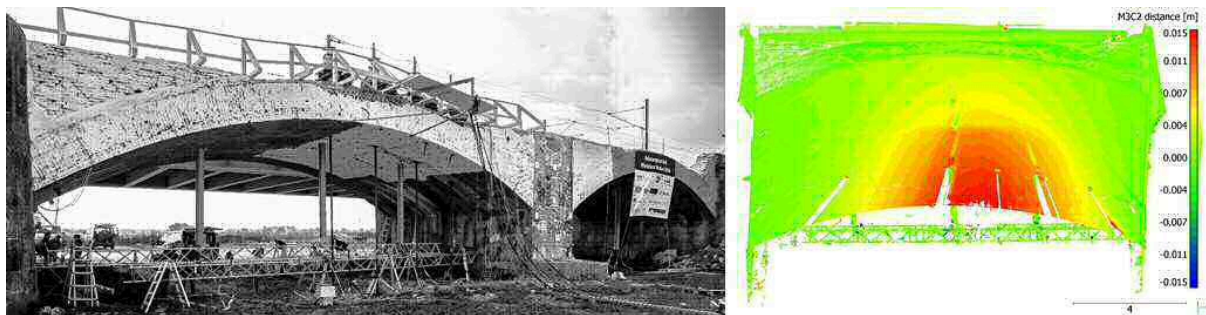
Fig. 4.1.3-1 Side view from West of the arch under investigation of the historic masonry arch bridge. The whitewashed area indicates the area of the direct influence of the load application. On the bridge: four hydraulic cylinders for the load application (left), 3D point cloud to 3D point cloud differences (M3C2) for the load scenario of 5 MN. Clearly visible is an arch displacement of up to 14 mm. [Paffenholz & Wujanz, 2019] (right)
